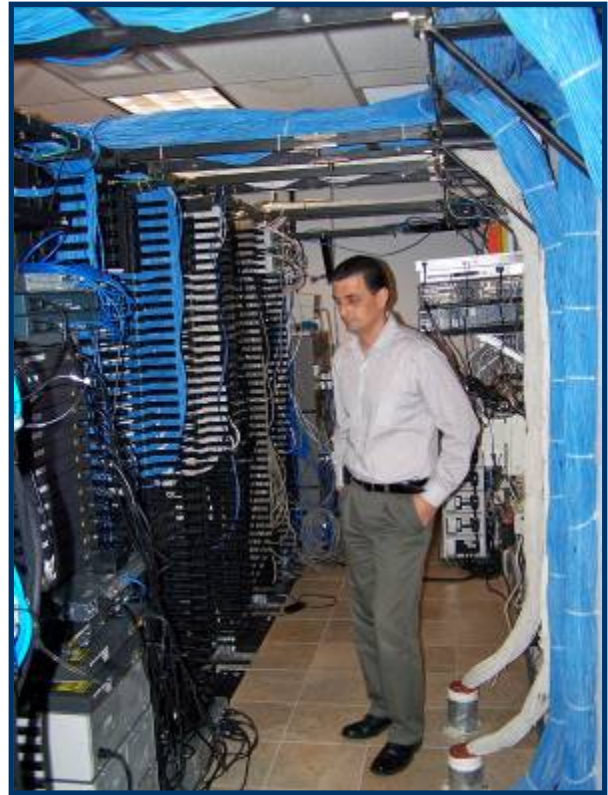
Eddie Mustafa, Systems Manager, shows off the professional level of installation and cabling FFP has accomplished in their Computer Center
